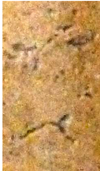
Fig. 20: Voids in the compacted sand
